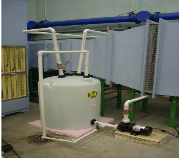
Figure 14: Heat exchanger cooling water pump and tank installation (Barbot 2003).
